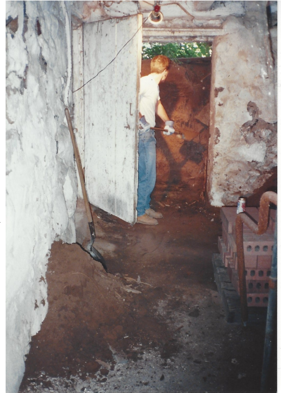
Whitewash on the fieldstone walls in the basement of the Bruentrup barn at the old location on White Bear Avenue during construction of a new wall.
