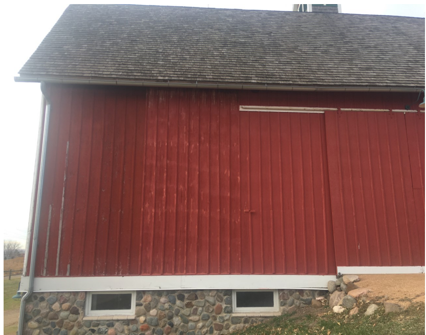
The left side of the Bruentrup barn wall has the old paint, the middle section has one coat of new red stain and the right side has two coats of red stain.
