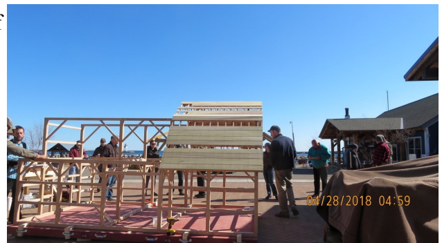
First assembly of the FoMB 1:5 scale model barn at North House School in 2018
